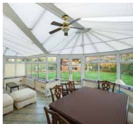
BEFORE the transformation with a tired polycarbonate roof.
